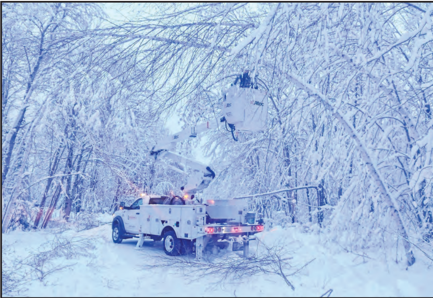
NCP Linemen, Seth Coggins and Paul Zmuda work through the tangled mess on Lagoon Road in Winter. The trees are so compromised by the weight of snow and ice, in many cases after the power has been restored another branch will fall and take it out again. This scene is indicative of what has occurred all over Sawyer County and what exactly these workers are up against. -Photo Courtesy of Paul Zmuda
